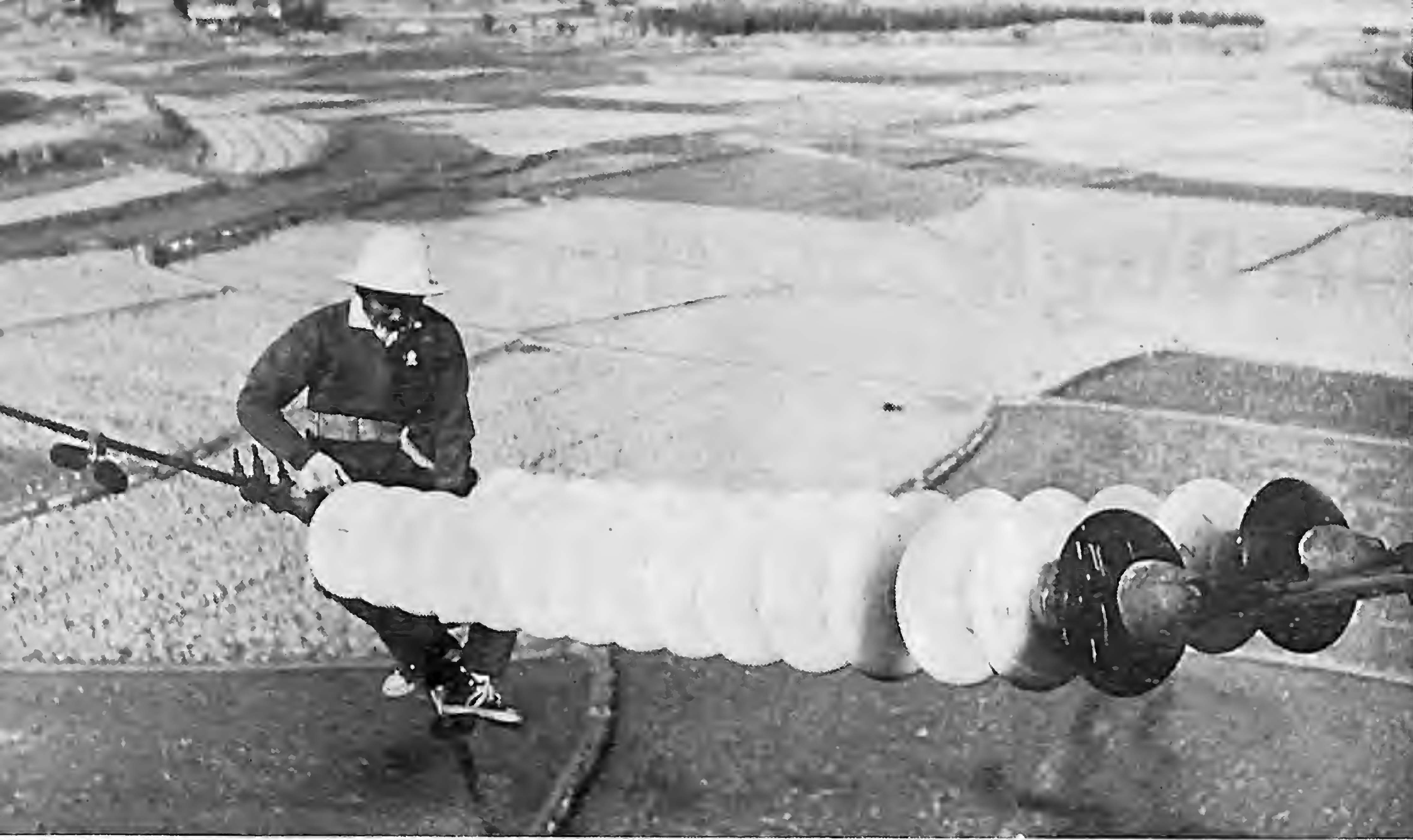
A woman from the Kwangchow (Canton) Power Company does maintenance work on a live ultra-high-tension power line.
